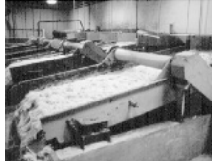
Four Link-Belt® Model NRM liquid Vibrating screens dewatering feathers and offal in a chicken processing plant.
