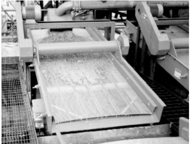
Single-deck NRM dewatering screen at a fish hatchery.
